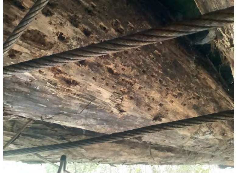
Stringer 11 dry rot, 1.5m inside bearing left bank
