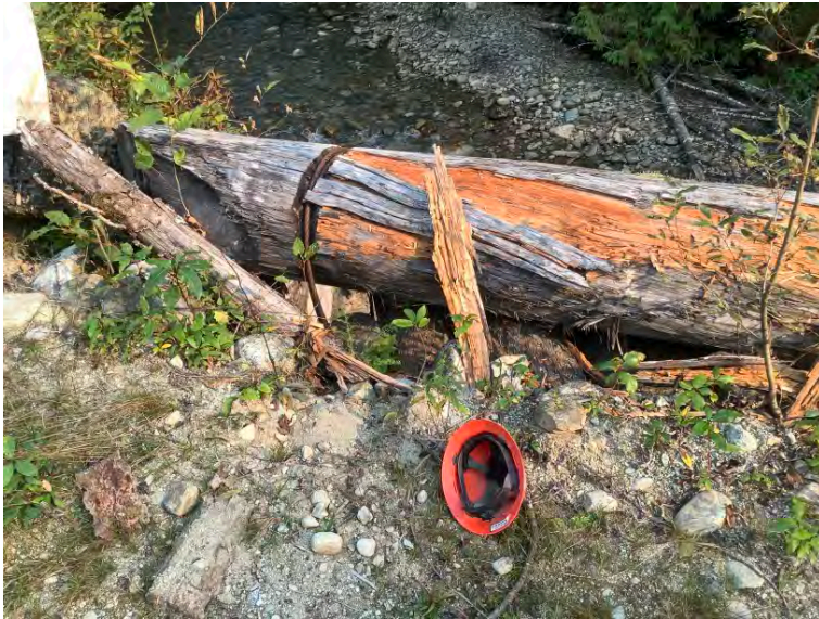
Material loss beneath curb log.
